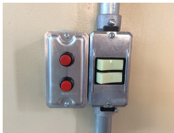
Figure 18. Buttons installed in the laboratory for user activation
