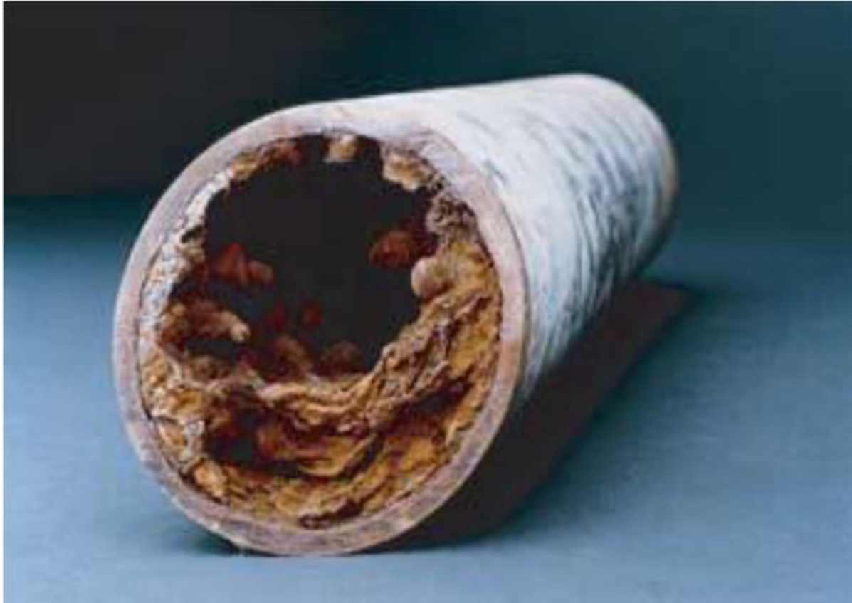
Fig 2.2 Oil Pipeline affected by Corrosion
