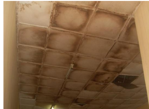
Plate 4: Rotten Ceiling due to roof leakages at Rumueme
