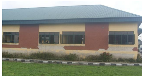
Plate 6: Riffed off Wall Tiles at Rumuwoji
