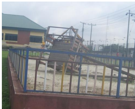
Plate 3: Damaged Recreational Facilities at Kpitem
