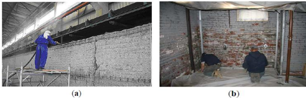
Fig.10. Shotcrete repair: (a) Concrete wall in factory; (b)Clay masonry walls (Augenti et al 2013).
